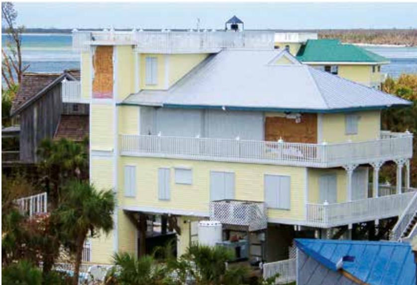
After Hurricane Charley, FEMA noted no structural damage to new wood-frame buildings built to the 2001 Florida Building Code standards.
